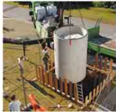
Installation des 1. KES-Speichers am ISFH (Sommer 2009)
